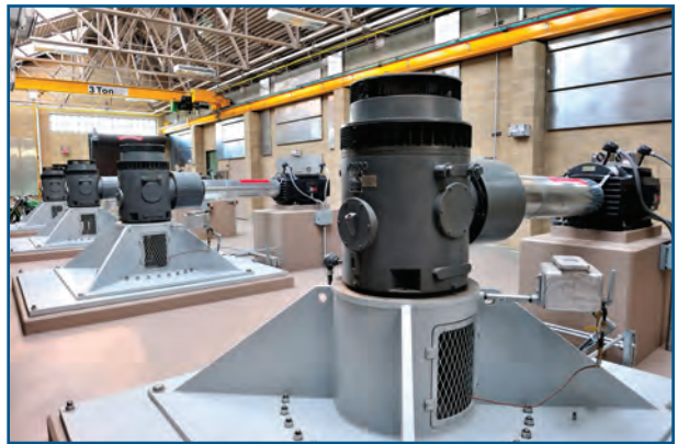
Horizontal Motor to Gear Drive
