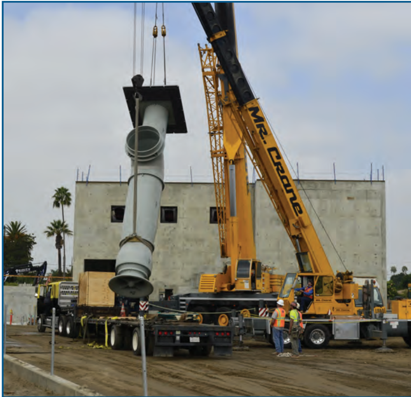
95,000 GPM STORM WATER PUMP
