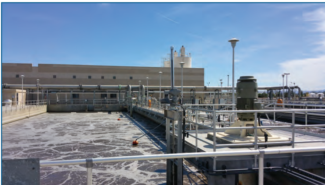
RETURN ACTIVATED SLUDGE (RAS)
